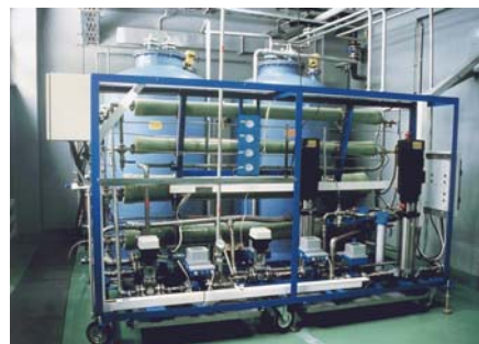
3-stage reverse osmosis installation
